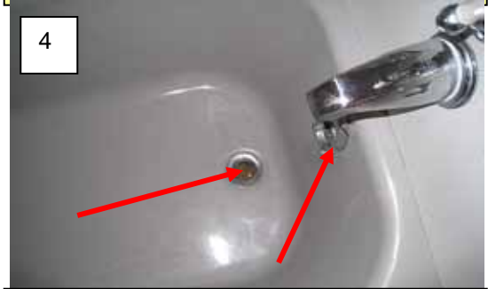
Item 19 - Strainer is busted out and stopper assembly is not working.
