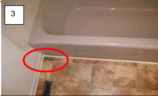
Item 29 - Floor is soft adjacent to ends of the bathtub.
