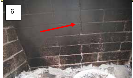
Item 23 - Open thermal cracks in the back of the firebox.
