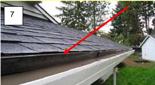
Item 2 - Drip edge flashing unfastened.
