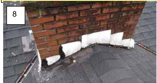
Item 1 - Chimney is improperly flashed in.
