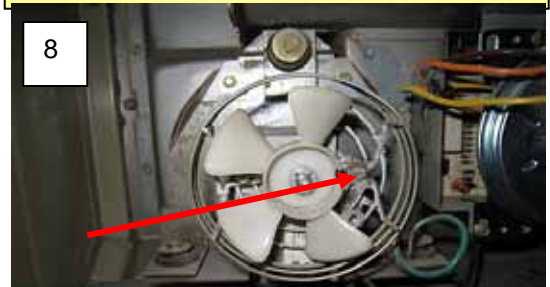
Item 21 - Fan blade broken off on exhaust inducer in the furnace.
