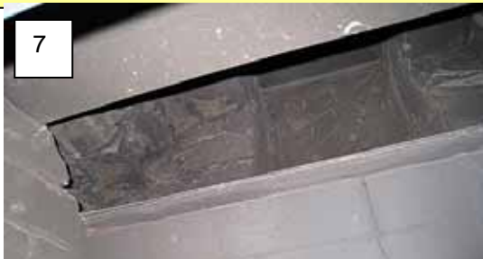
Item 23 - Damaged damper and throat of the fireplace/chimney.
