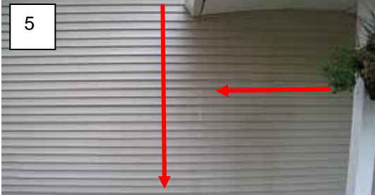
Item 7 - Water streaming down from gutter interface siding on the left side of the front entry.
