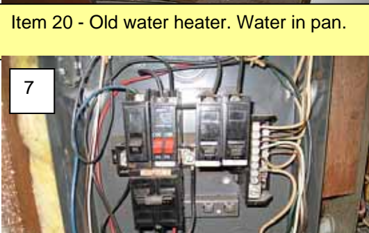
Item 12 - No proper 4 conductor feeder to sub panel. No isolation of grounds and neutrals.
