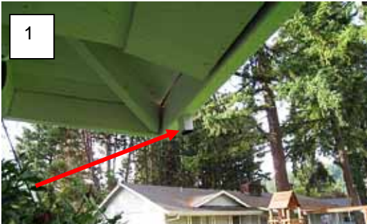
Item 2 - Missing downspout on the front entry.
