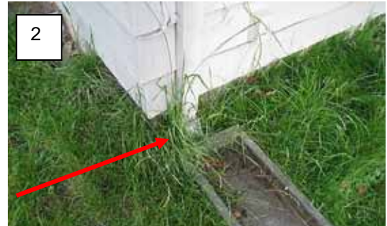
Item 2 - Downspouts drain next to the house.
