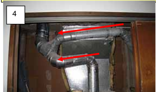
Item 21 - Item 20 - Furnace and water heater vents slope downwards.
