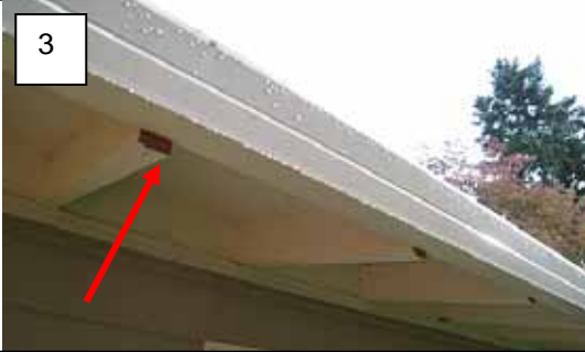
Item 6 - Rafter tails are not painted at their ends.
