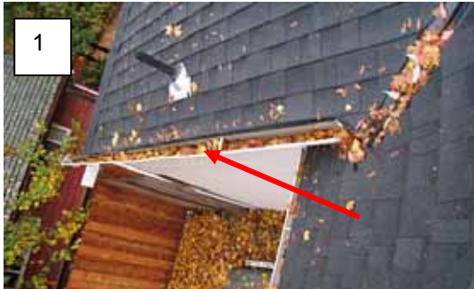
Item 2 - Gutters need cleaning.
