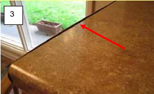
Item 28 - Protruding end cap on kitchen counter is vulnerable to damage.
