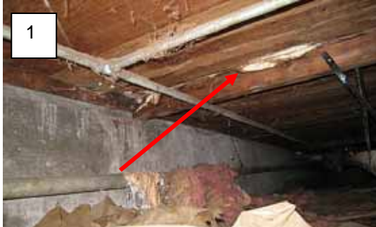
Item 29 - Heavy moisture stains, decay fungi, and rot damage to floor under bathtub.
