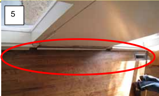
Item 19 - Moisture deterioration to wood flooring along the south wall in the living
