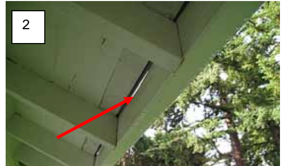
Item 2 - Gap between the roof and gutter on the front of the house.
