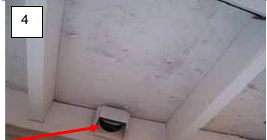
Item 27 - Bathroom vent housing not mounted right. Damper door is always open.
