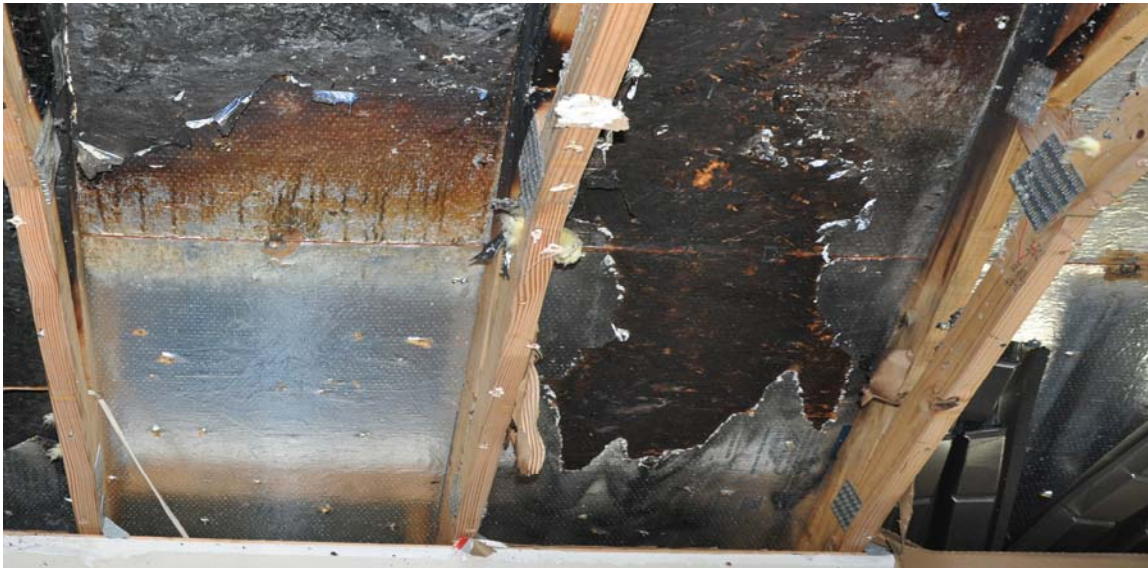
Photo # 12 Photo from an Actual Attic Fire After a Confirmed Lightning Strike
