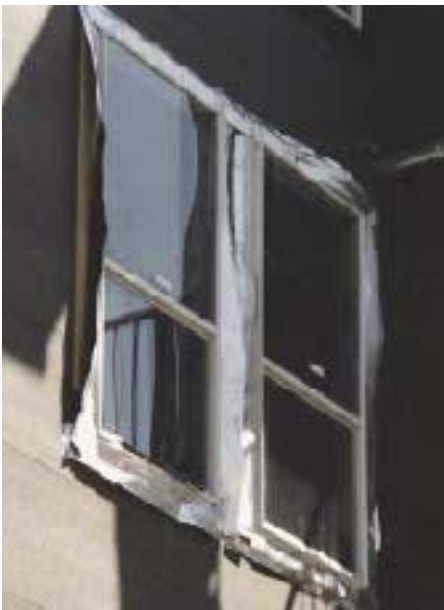
Figure 8. Peel-and-stick flashing adheres poorly to dirty substrates or when applied in cold weather.
