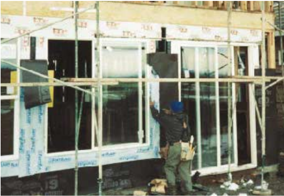
Figure 7. Builders use a variety of methods for flashing windows. This installer has chosen a belt-and-suspenders approach, installing strips of FortiFlash, a rubberized-asphalt flashing, on top of strips of E-Z Seal, a kraft-paper flashing laminated with polyethylene and fiberglass reinforcement.
